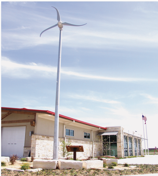
Residential wind turbine at the Seguin Office Complex.
